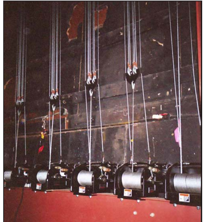
A row of Thern clew winches hold set lines in place at the Diamond Head Theatre.
