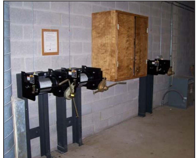
Thern clew winches installed at the Phillippe Center.
