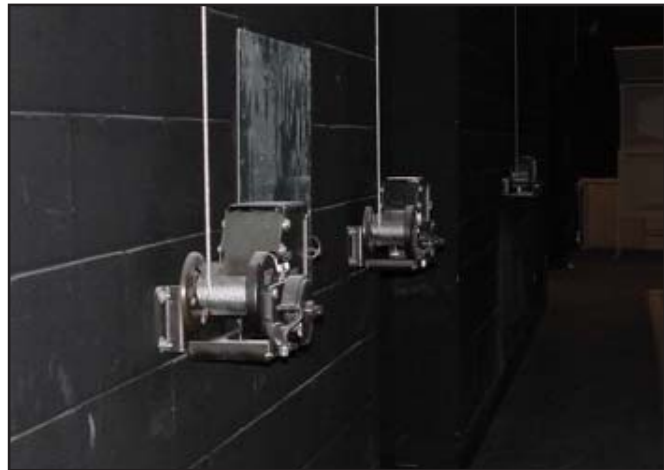
Thern FVC winches installed along the wall backstage.
